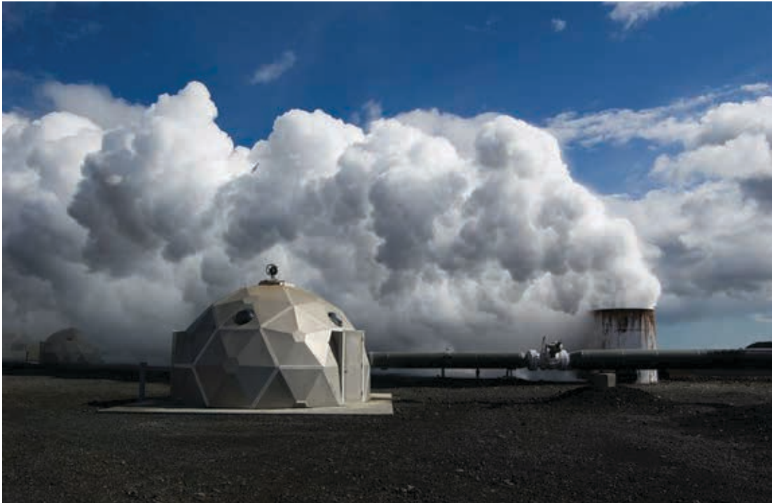
FIGURE 2.4 Geothermal Well Head and Silencer
